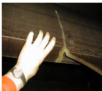
Figure 2: Fatigue crack on stiffener [1].
